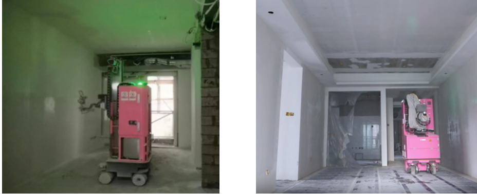
Figure 1: Typical indoor working conditions for construction robots (Figures are from Bright Dream Robotics(BDR) company in Foshan, China, which provides us the building sites for data collecting.)
